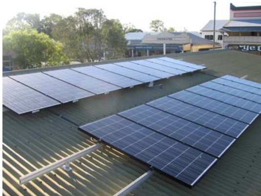
Figure 4 – Solar Panels on Gordonvale Library
