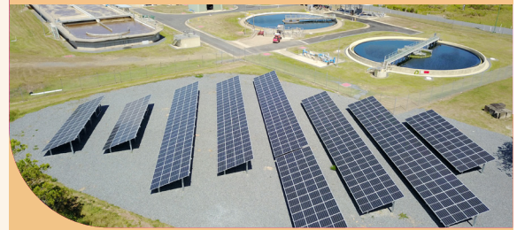
Ground mount solar PV system at Northern Wastewater Treatment Plant
