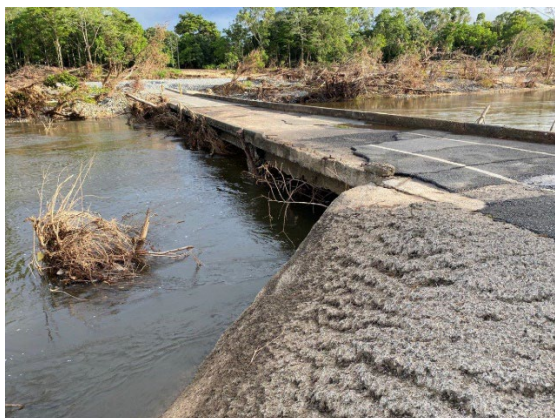
Lower Kamerunga Cycleway: view from southern abutment, facing north, showing loss of asphalt running surface, damaged kerb and beams.
