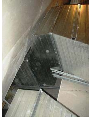
Figure 7 Poor Duct Elbow Geometry
