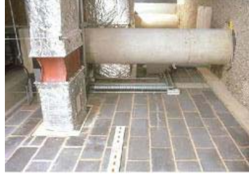
Figure 8 Flexible duct connection and sealed penetration at an isolation joint
