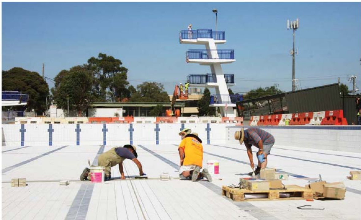
Photo 9 – 50m Outdoor lap pool under construction at the Monash City Council's Oakleigh Aquatic & Recreation Centre
