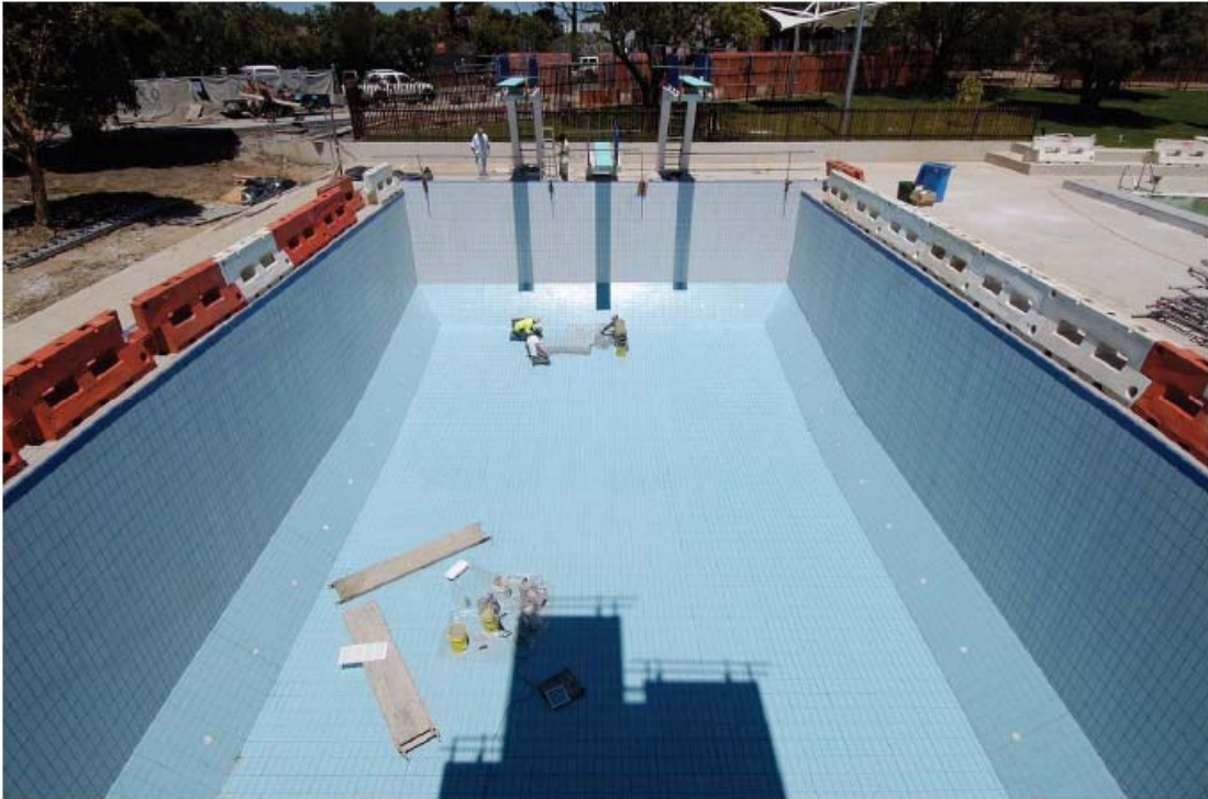
Photo 8 – 5m deep Diving pool under construction at the Monash City Council's Oakleigh Aquatic & Recreation Centre
