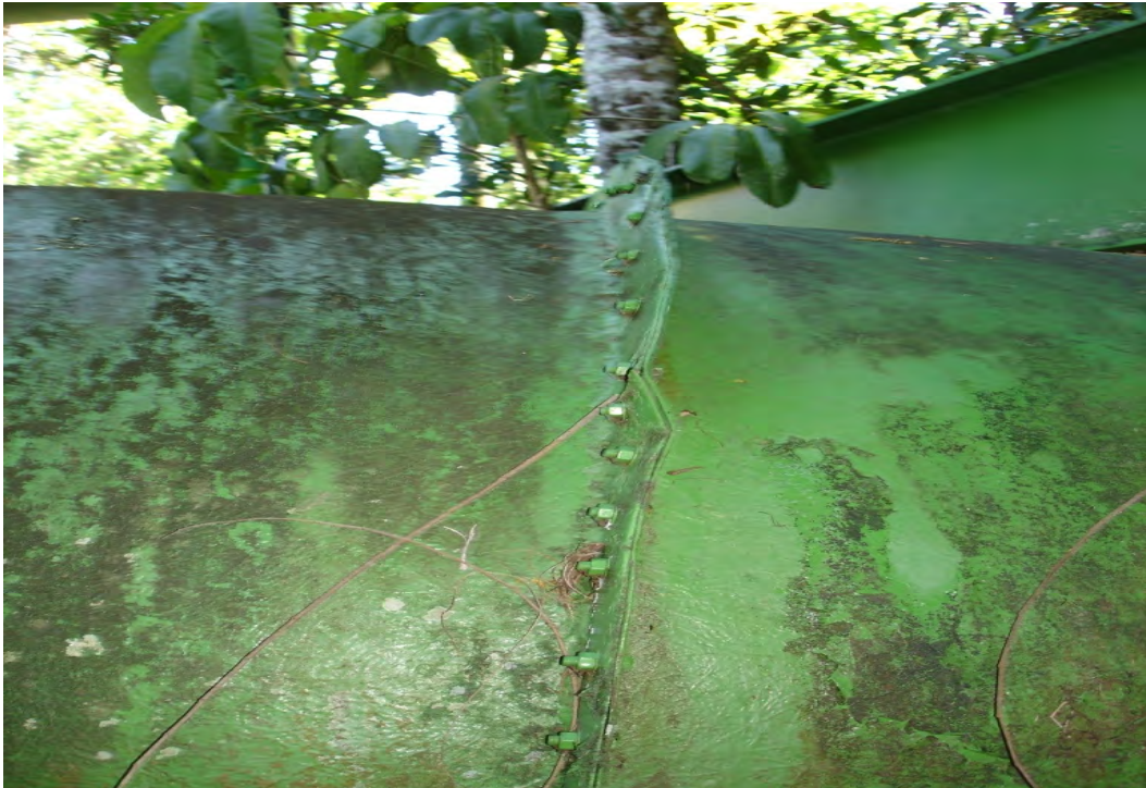
5. Vertical tubing flange joints buckling
