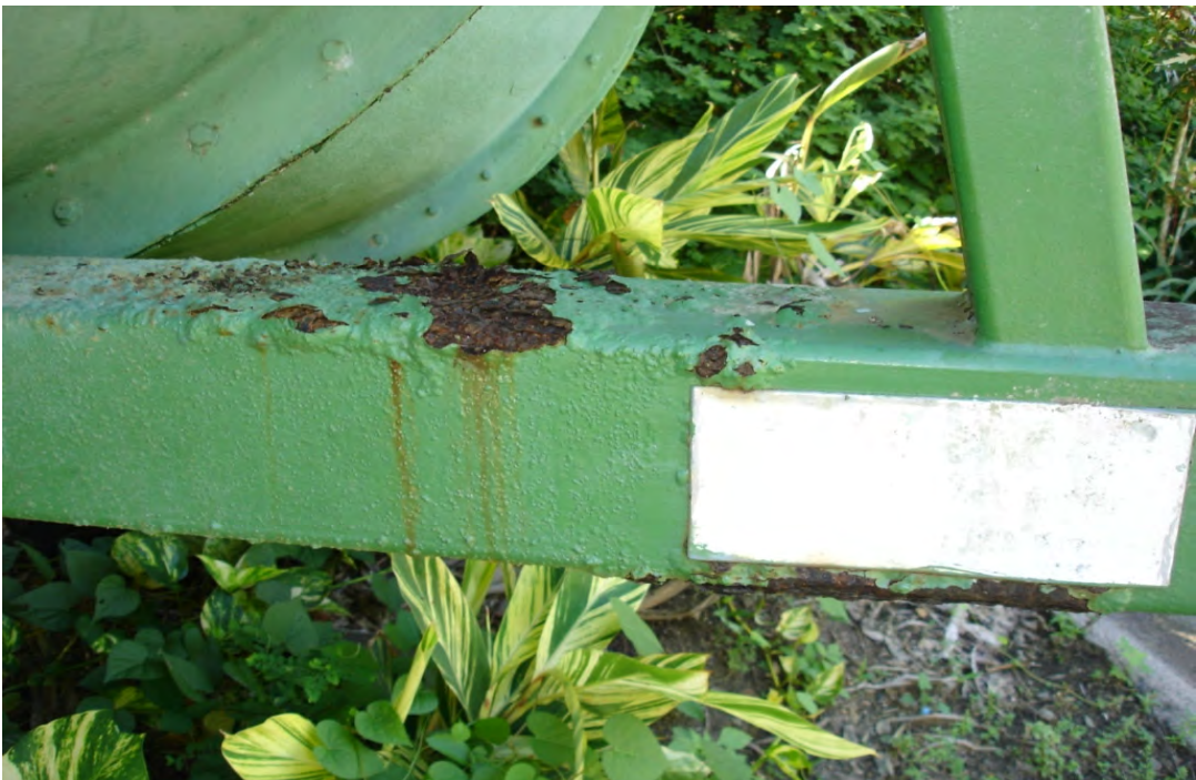
10. Steelwork rusting to Flying Fox waterslides
