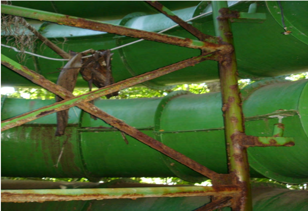
9. Corroded steel frame supporting tubes for The Cyclone waterslide
