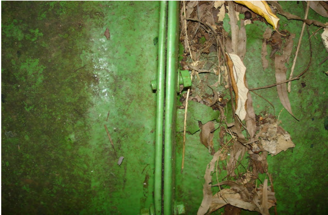
11. Missing bolt nut
