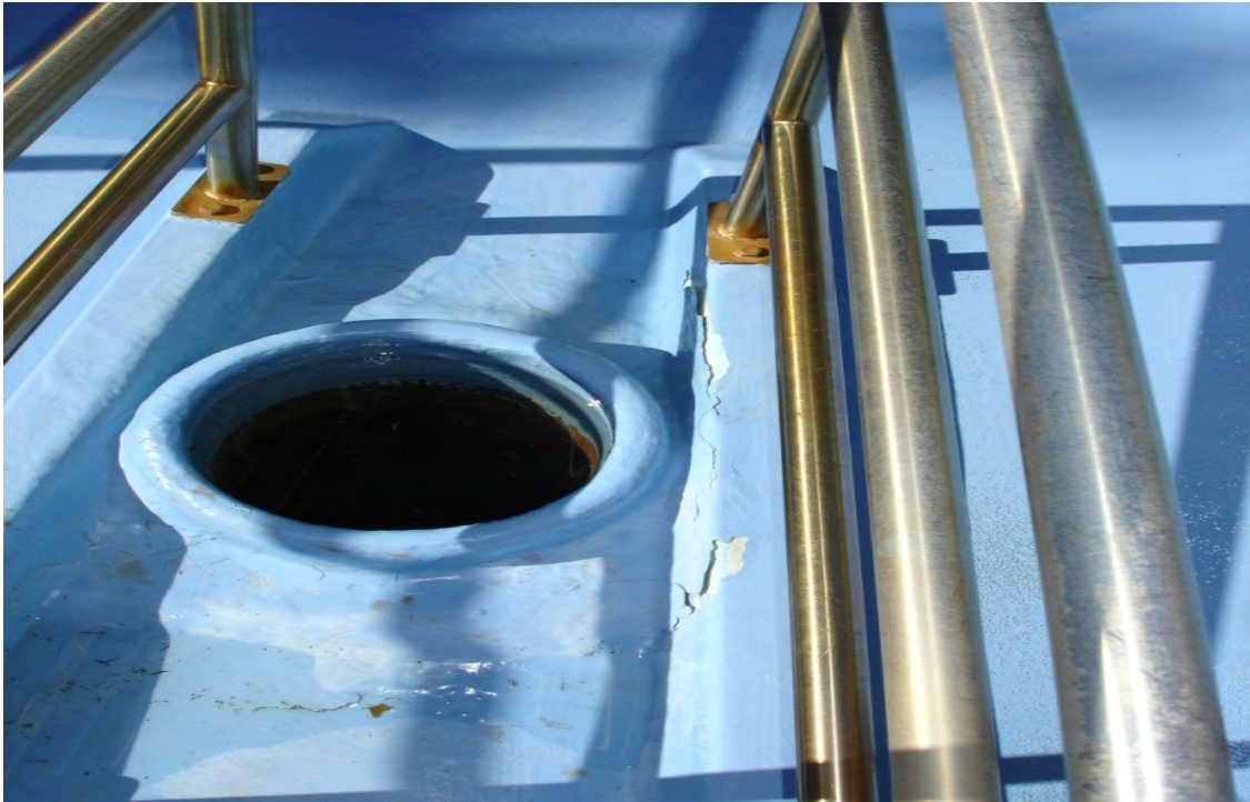
13. Cosmetic delamination of paint finishes near waterslides entry
