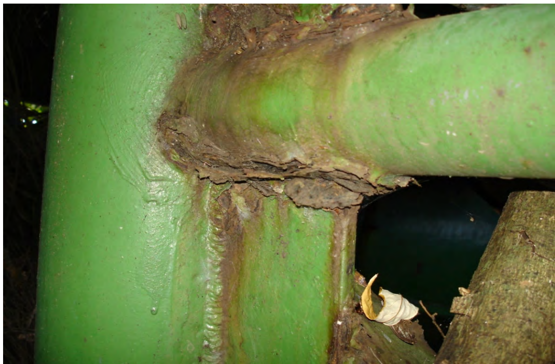
8. Corroded steel tubes for The Cyclone waterslide
