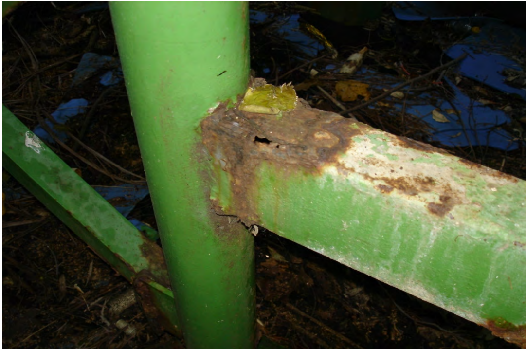
7. Severely rusted steelwork for The Cyclone waterslide
