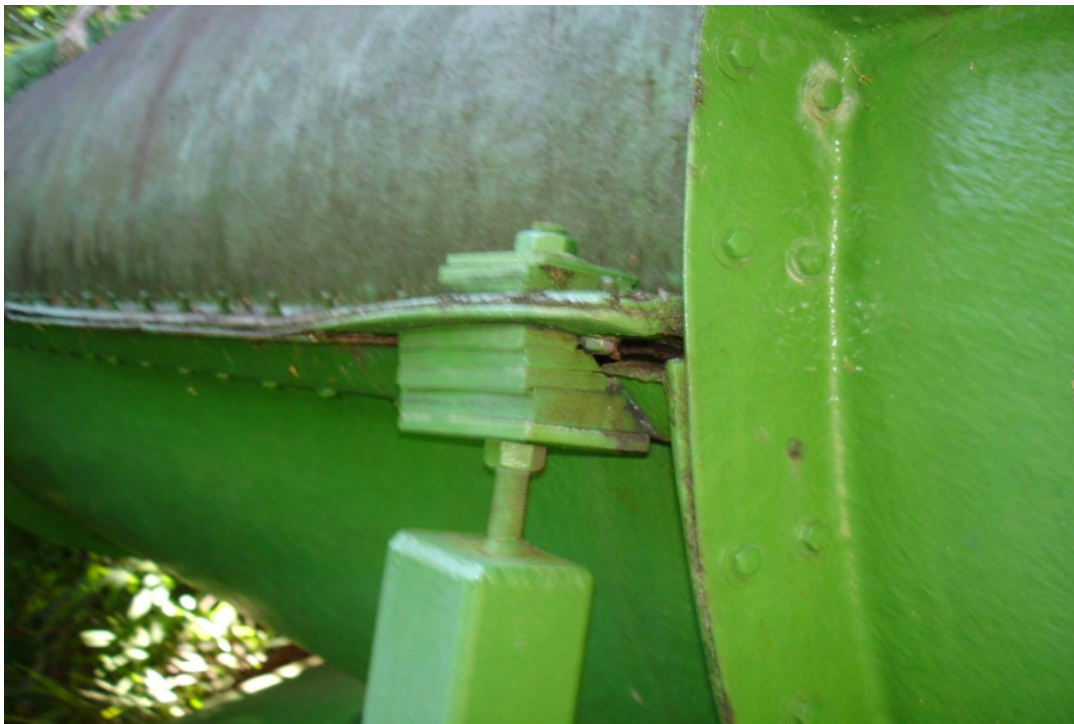
6. Flange joints cracking and buckling at support locations
