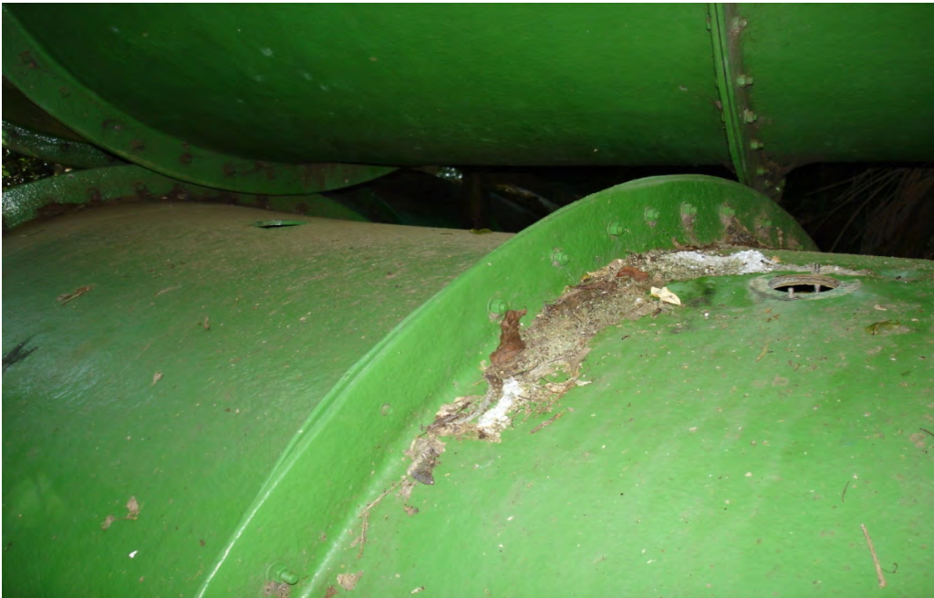
4. Holes to top of tubing at missing lights
